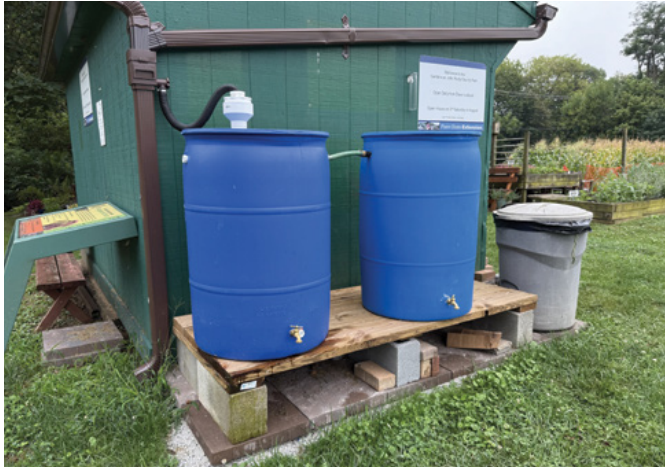
Figure 28a. Rain barrel connected to downspout via sealed diverter. (Jodi Sulpizio)
