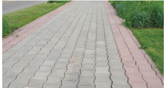
Figure 29a. Permeable block pavers infiltrate runoff before it flows onto the lawn or street. (Andy Yencha)
